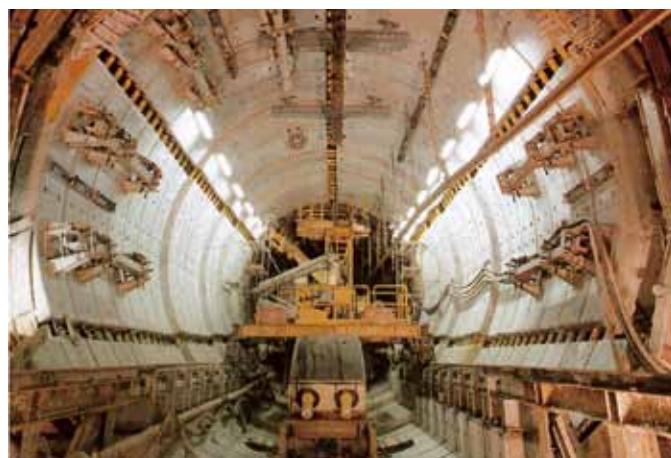
Fig. 4. Shaft landing with concrete segment supports and deformation elements (yellow row of props).
