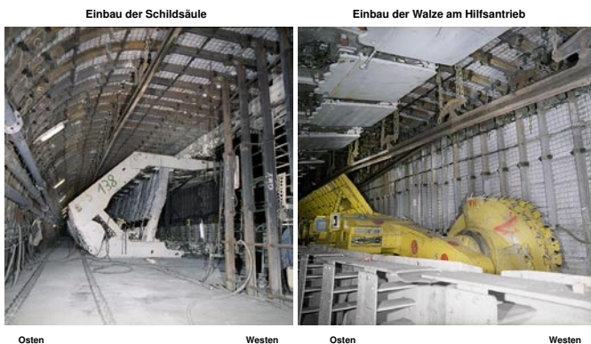
Fig. 15. Face start-up road 1238 – equipping phase (installation of shield line and coal shearer)
