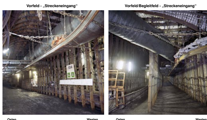
Fig. 14. Face start-up road 1238 – permanent supports in the advance heading and parallel drivage sections
