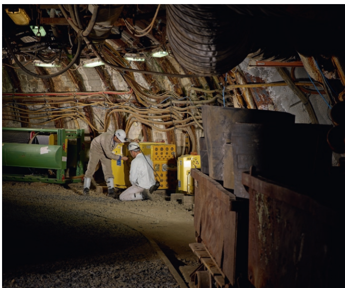
Fig. 1. The classic cable and looms used in mining are pushed to their limits in many areas and have to be reconceived if they are to fulfil the demands of the modern day.
