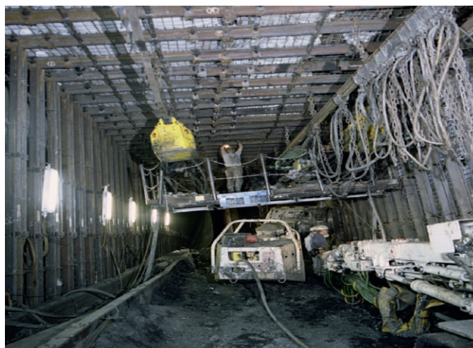
Fig. 3. First stage of the start-up heading with a floor width of 7.2 m.
