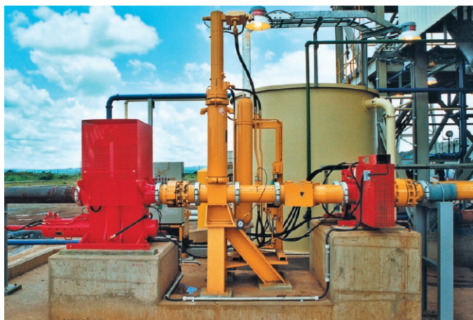
Fig. 9. Scraper pig gate; damper; gate valve (left to right).
