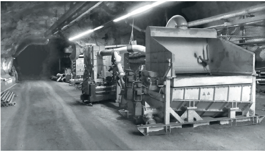
Fig. 4. Plant for pneumatic stowing in the old workshop drift 403 (4 th level).
