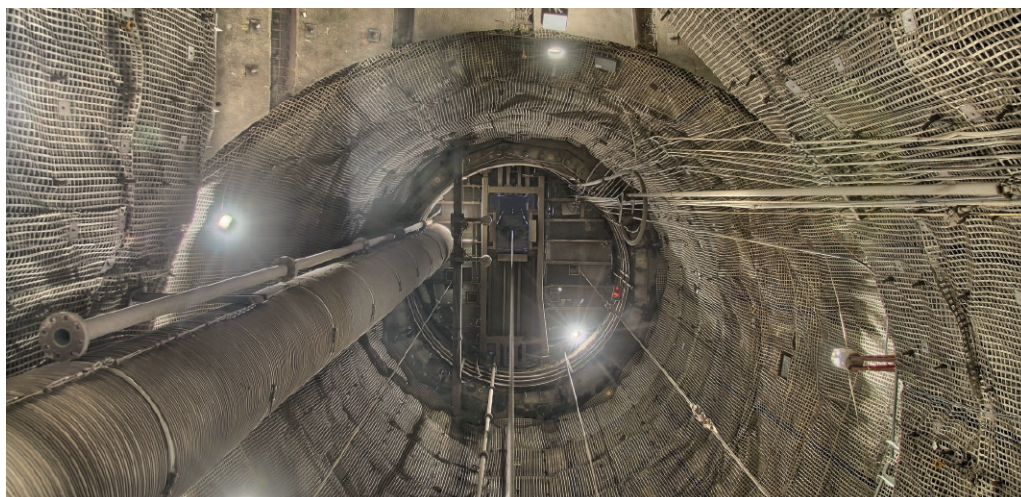
Fig. 2. Shaft Konrad 2 in the area of the extension between 840 and 875 m depth. View from the working platform to top.
