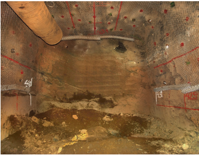
Fig. 1. View along the axis of a storage chamber with anchor and mesh wire retention at the time of excavation.
