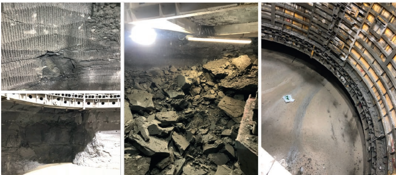
Fig. 11. Overbreak at Shaft 2 just underneath the freeze shaft, March 2019.
