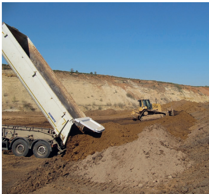
Fig. 2. Delivered and stock-piled soil material in an open-pit mine before external control and final integration.
