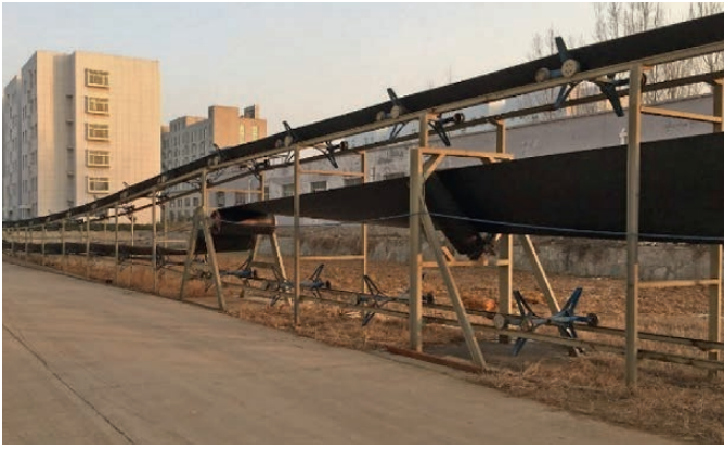
Fig. 4. Rail Conveyor prototype system operating in China. Bild 4. Rail Conveyor-Prototyp in Betrieb in China. Source/Quelle: tk
