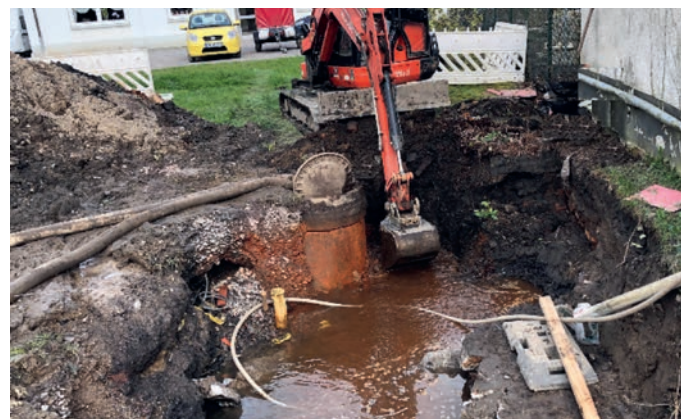
Fig. 3. Trench with exposed drainage shaft and water inflow.
