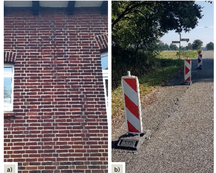
Fig. 2. Examples of mining-related damage: Gregor school in Bottrop-Kirchhellen (a), repairs to a cracked wall surface, Langer Weg (b), scarred road surface.
