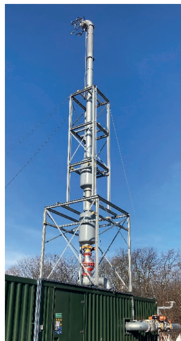
Fig. 3. Mine gas extraction system at the Centrum 2 shaft.
