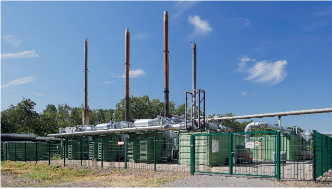
Fig. 6. Westerholt mine gas plant.
